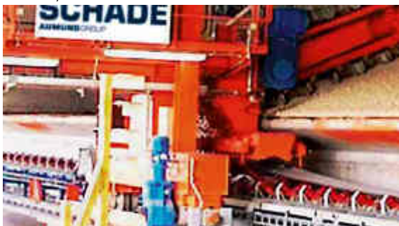
Discharge via impact idler table
