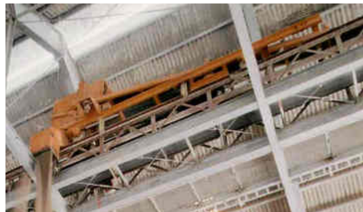
Fig. 5 Travelling tripper carriage
