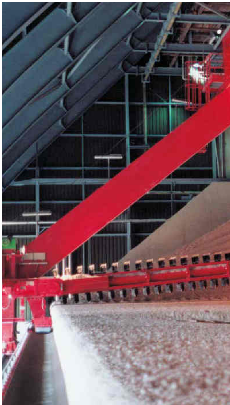
Portal Scraper Reclaimer, 32 m span, 400 t/h, FGD-Gypsum
