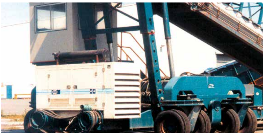
Combined Gen-Set and electric drive
