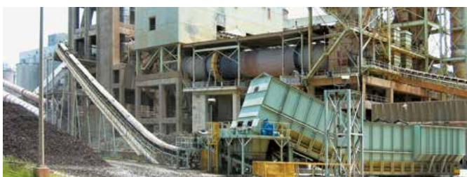
Output regulated by weigh belt feeder with belt conveyor onward transport
