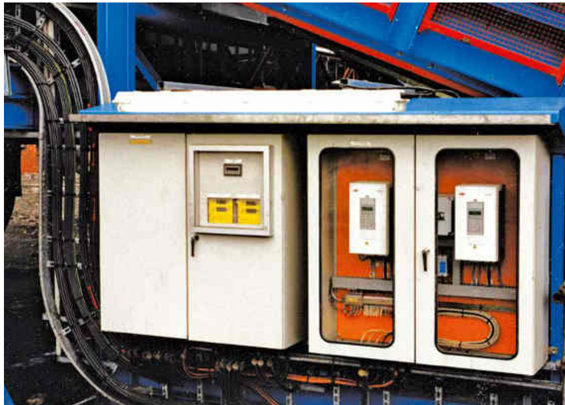
Inverter speed control modules located local to the Samson® Material Feeder but linked to a remote control room
