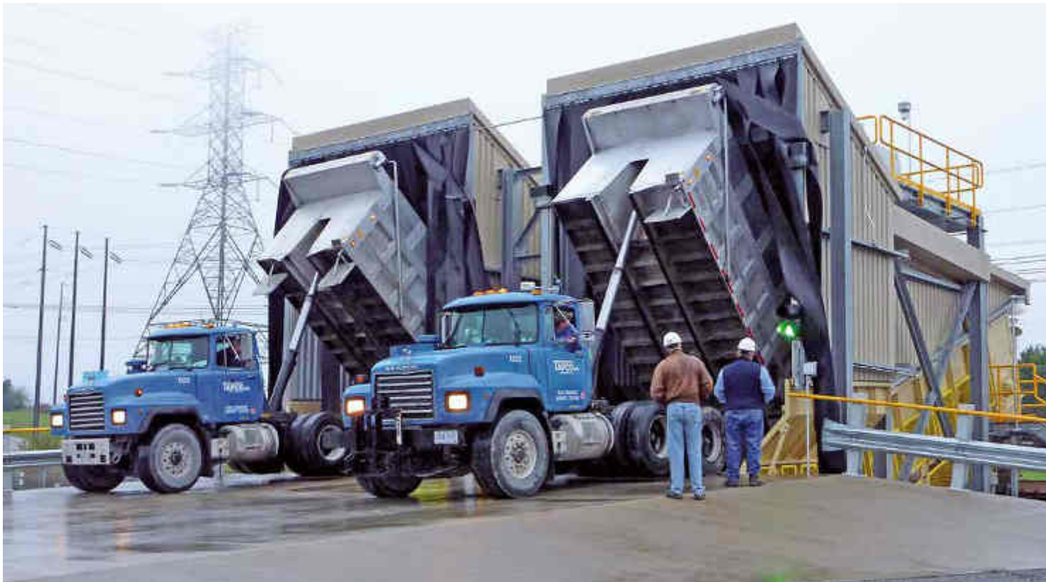
Twin Samson® Material Feeders receive minus 25 mm limestone for the flue gas desulphurisation system in an US American power plant
