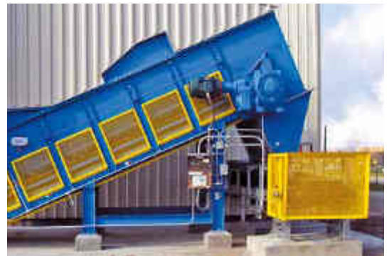
Synthetic gypsum discharged to horizontal belt conveyor
