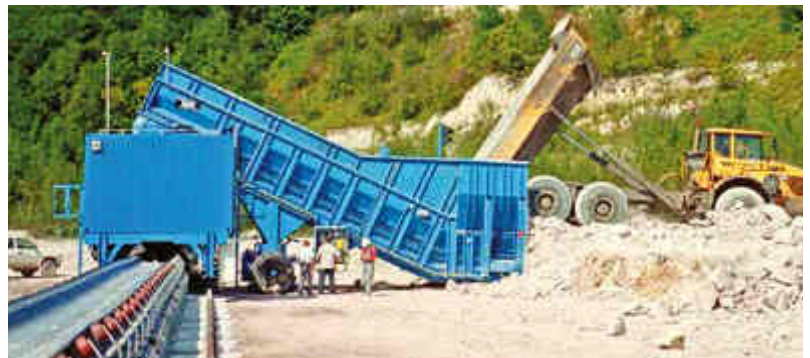
Mobile Samson® Material Feeder receives as-mined limestone from articulated trucks
