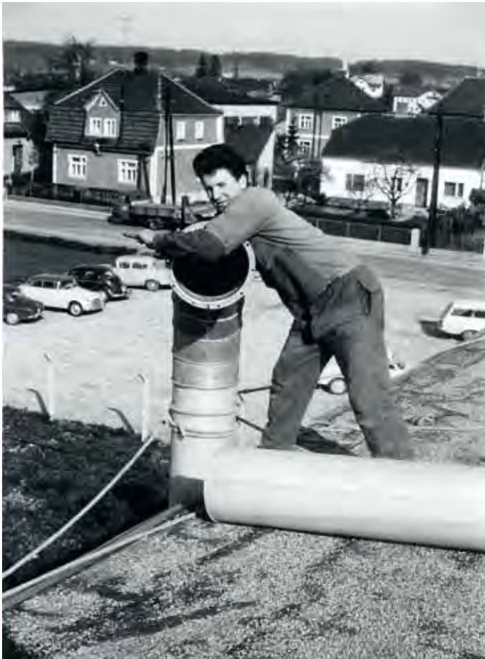
PIPING FOR A DEDUSTING SYSTEM MARKS THE FIRST STEP TOWARDS "TECHNOLOGY FOR CLEAN AIR".
