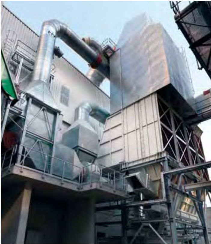
THE LEUBE CEMENT PLANT IN THE AUSTRIAN TOWN OF ST. LEONHARD COMMISSIONS A CLINKER COOLER DEDUSTING PLANT FROM SCHEUCH IN 2010.
