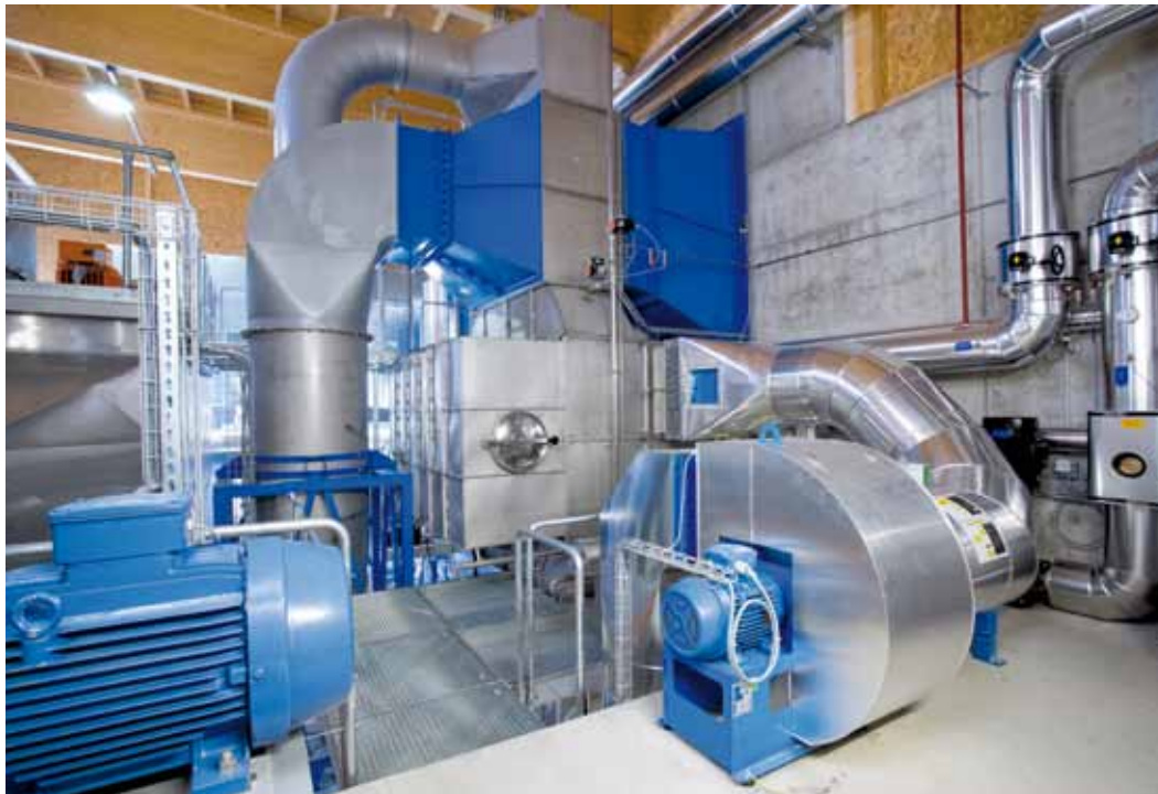
IN 2010 IN THE SWISS TOWN OF GRINDELWALD A FLUE GAS CLEANING PLANT WITH ERCS IS ERECTED.
