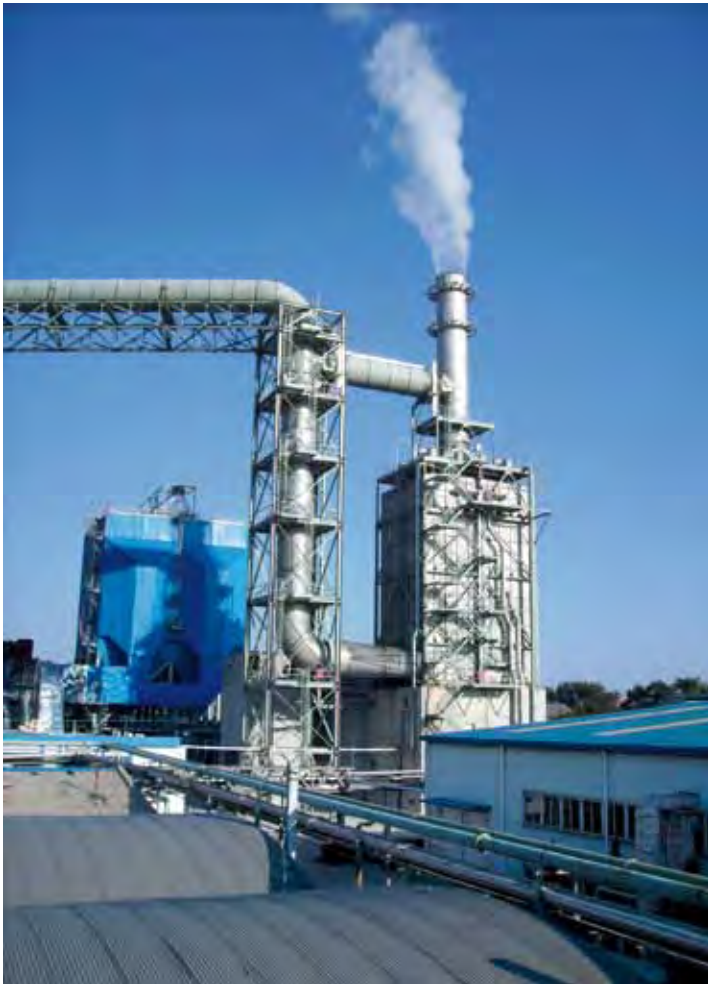
IN 2008 SCHEUCH BUILDS A BIOSENA PLANT FOR KRONOSPAN IN PEKING.
