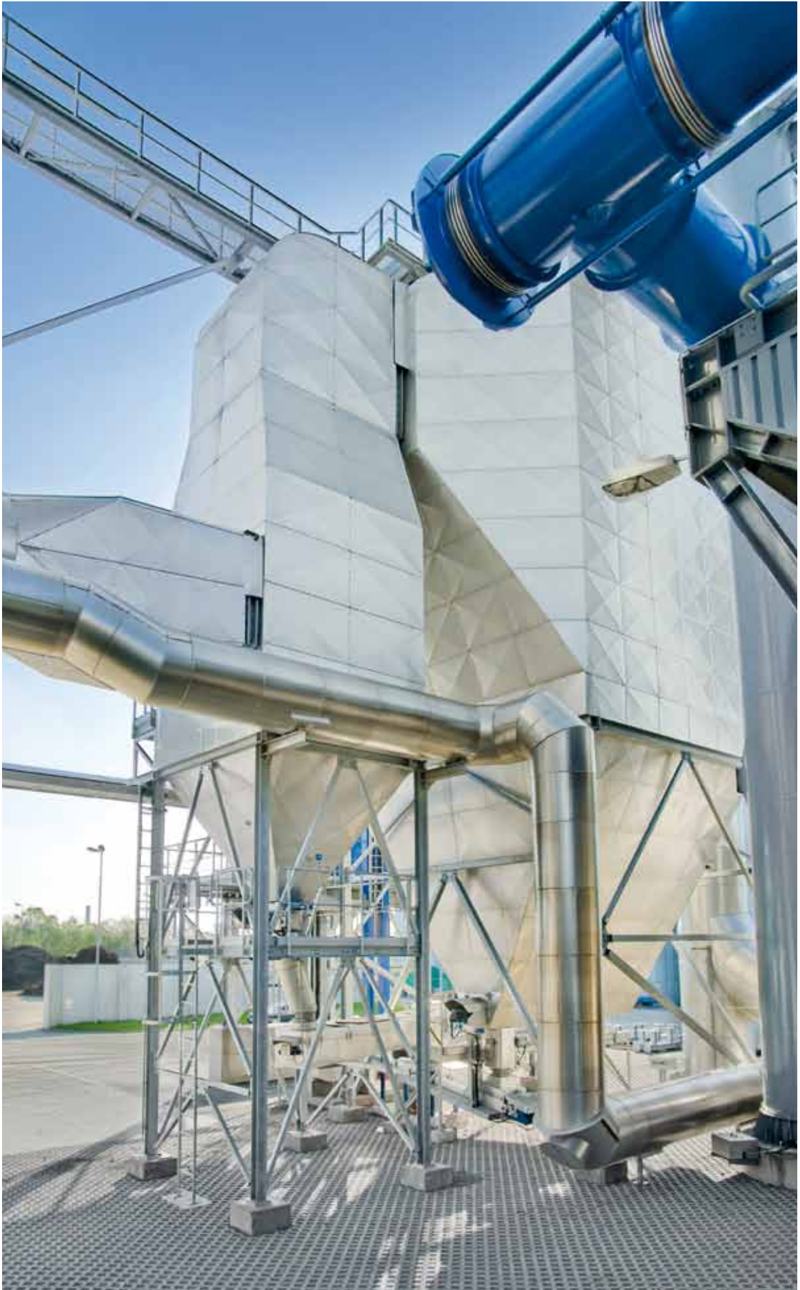
PARTICULATE COLLECTION FOR THE WITTGENSTEIN BIOMASS HEAT AND POWER GENERATING STATION IN ERNDTEBRÜCK, GERMANY, COMMISSIONED 2009.
