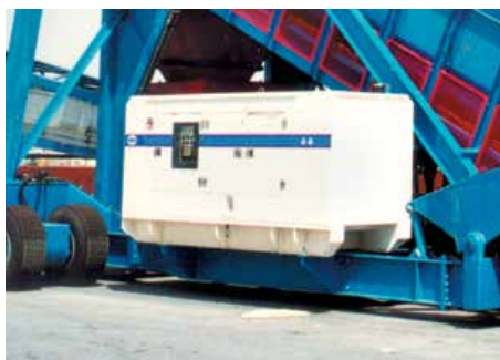
Diesel Gen-Set mounted to the main chassis within a sound attenuated enclosure
