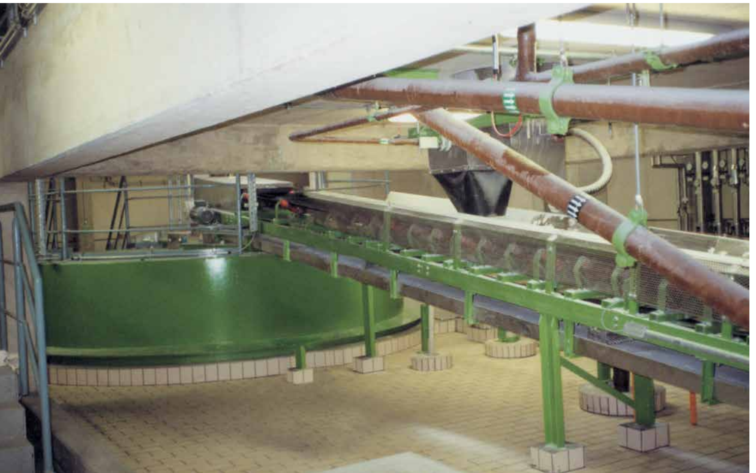
CENTREX™ - Feeding of FGD Gypsum to silo
