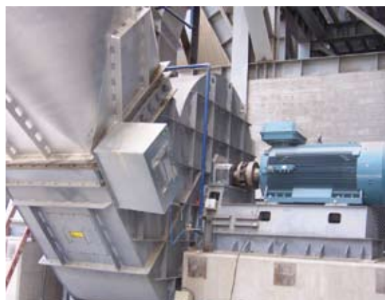
Process fan with double-sided bearings
