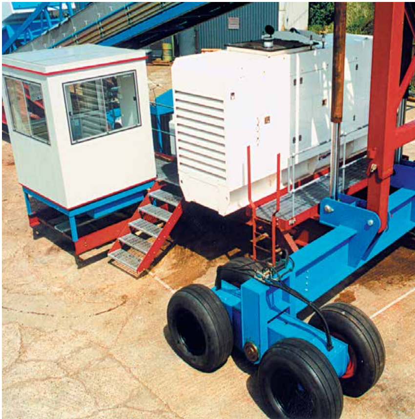
Diesel Gen-Set drives the complete Shiploader and Feeders
