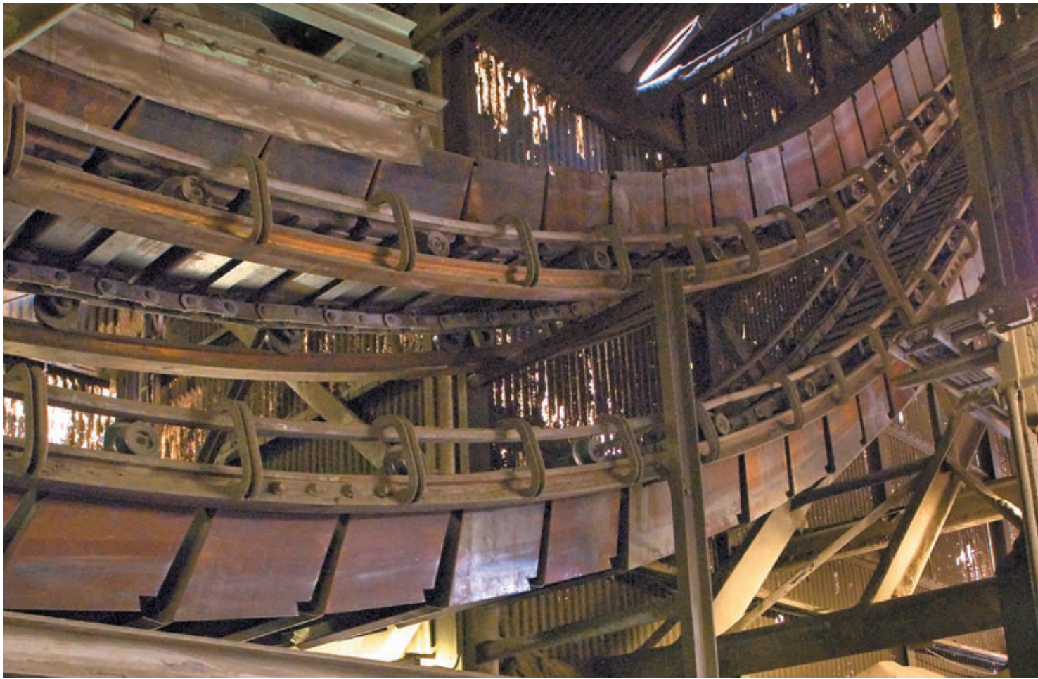
Bucket Apron Conveyor
