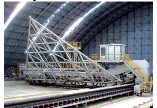
SCHADE bridge reclaiming for output homogenisation
