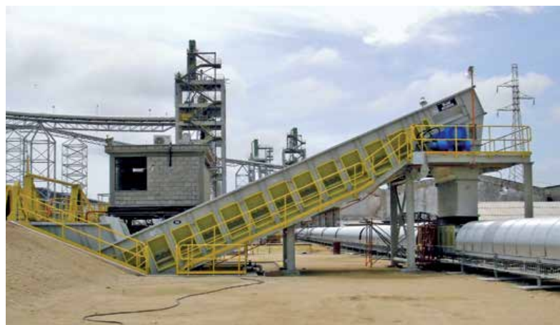
Samson™ discharges directly to overland conveyor
