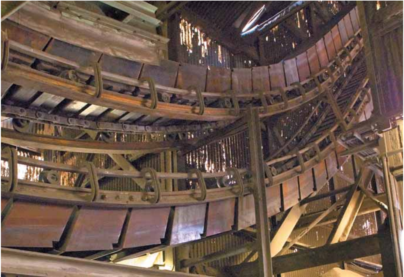
Bucket Apron Conveyor
