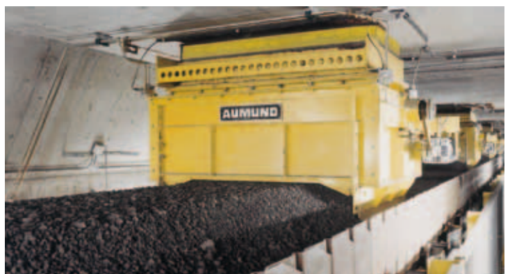
Gravity silo discharge
