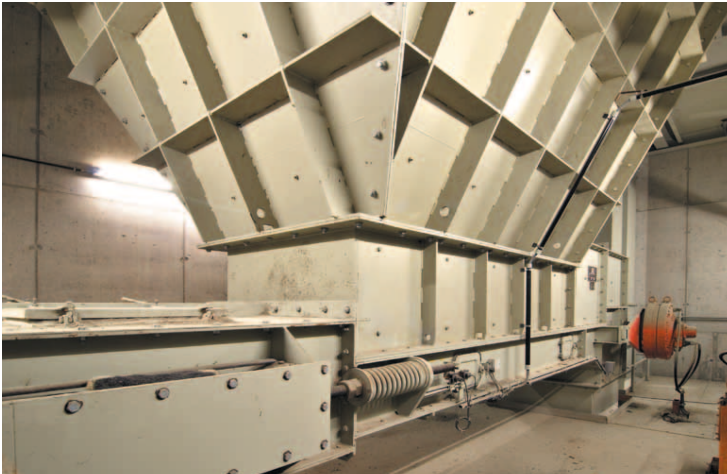
Hopper discharge with Armoured Chain Conveyor
