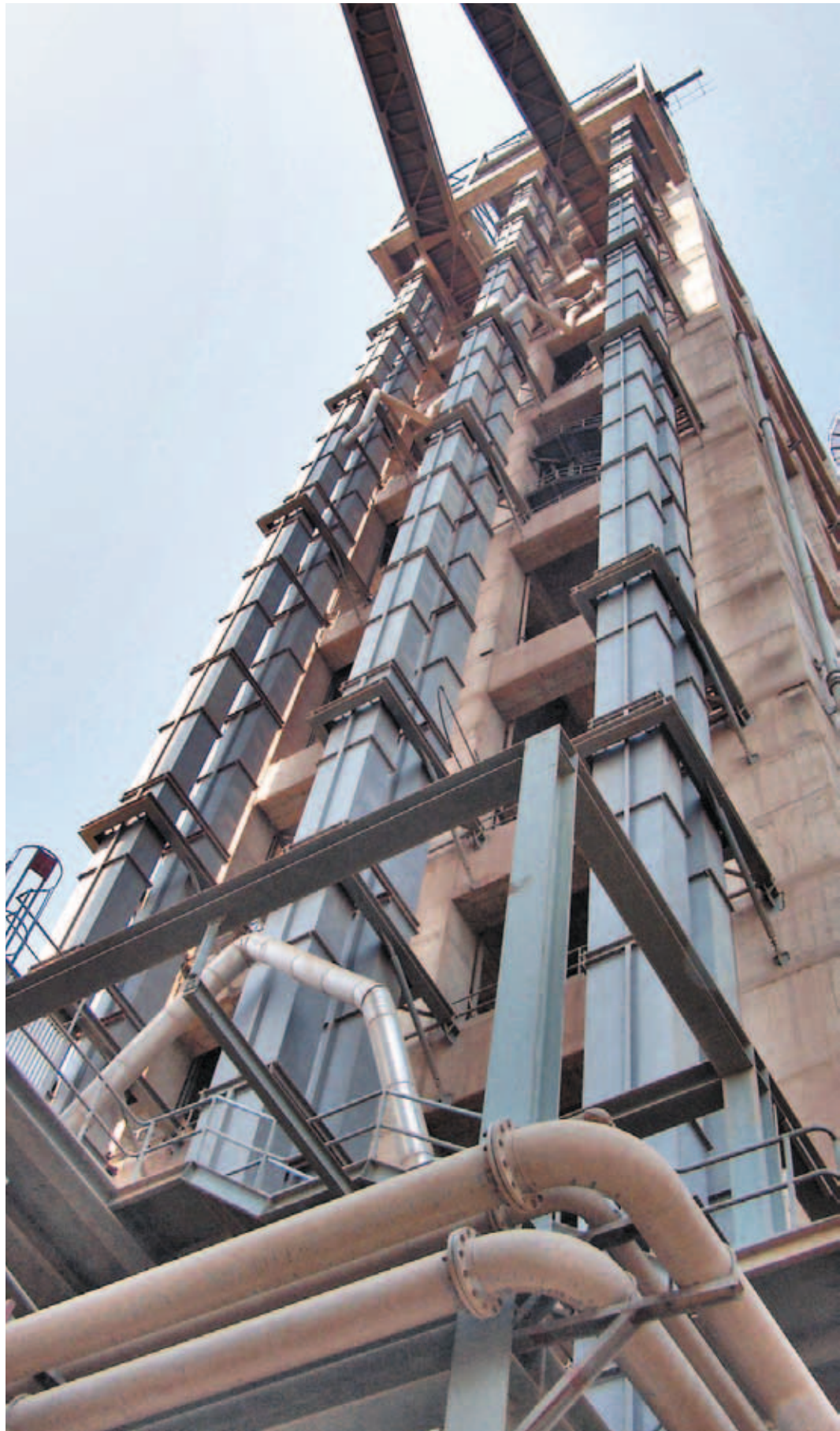
Belt Bucket Elevators handling raw meal
