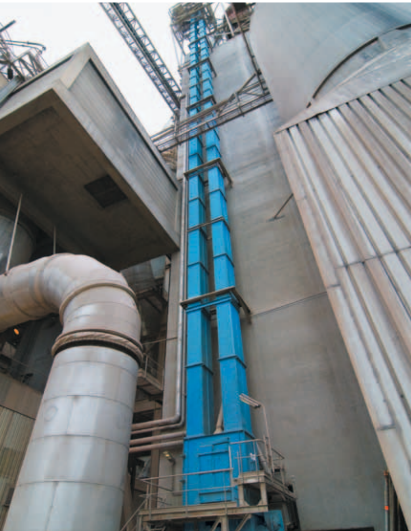
Bucket Elevator for silo feeding
