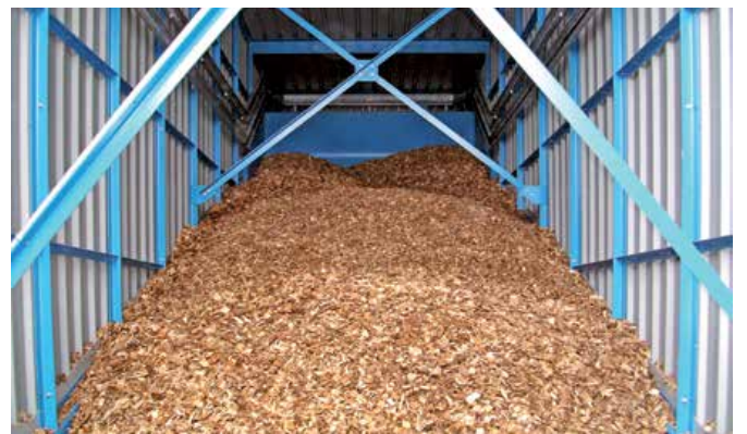
Wood Chip Intake for a Brewery Steam Boiler
