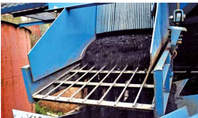
Vibro-Feeder with reject grill to remove over size material
