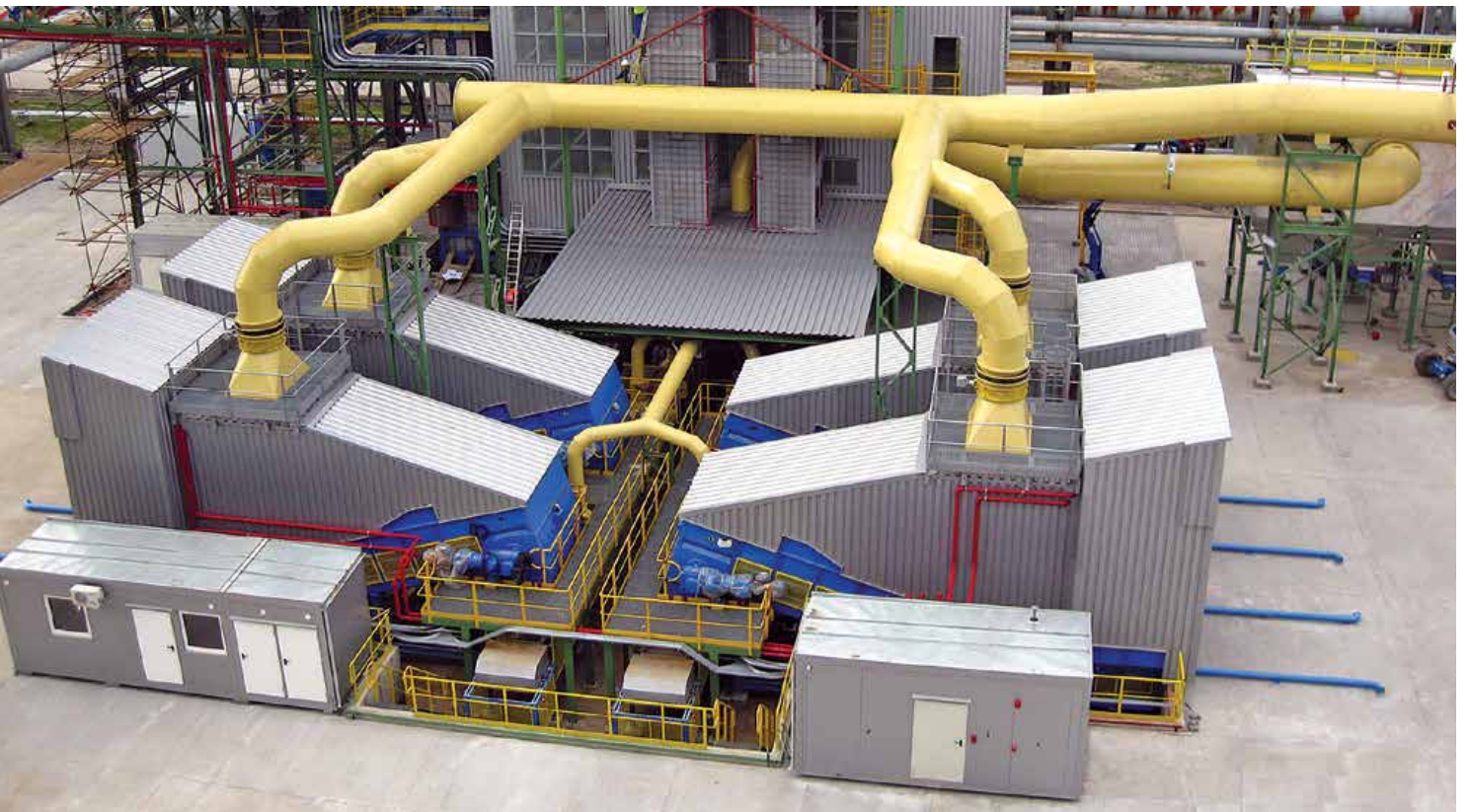
Four Samson™ Material Feeders provide an Alternative Fuel Intake facility to a major Power Plant
