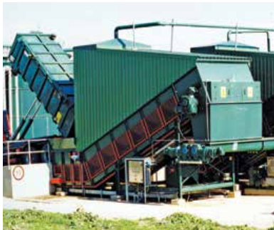
Enclosure with fume extraction for odious materials
