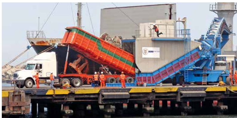
Samson™ Material Feeder integrated to a Mobile Shiploader receives Copper and Gold concentrate
