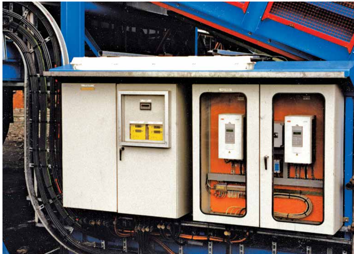
Inverter Speed Control Modules located local to the Samson™ Material Feeder but linked to a remote control room
