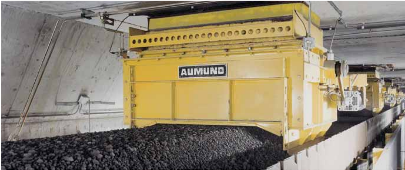
Silo Discharge by Remote Control – Discharge Capacity 750 t/h
