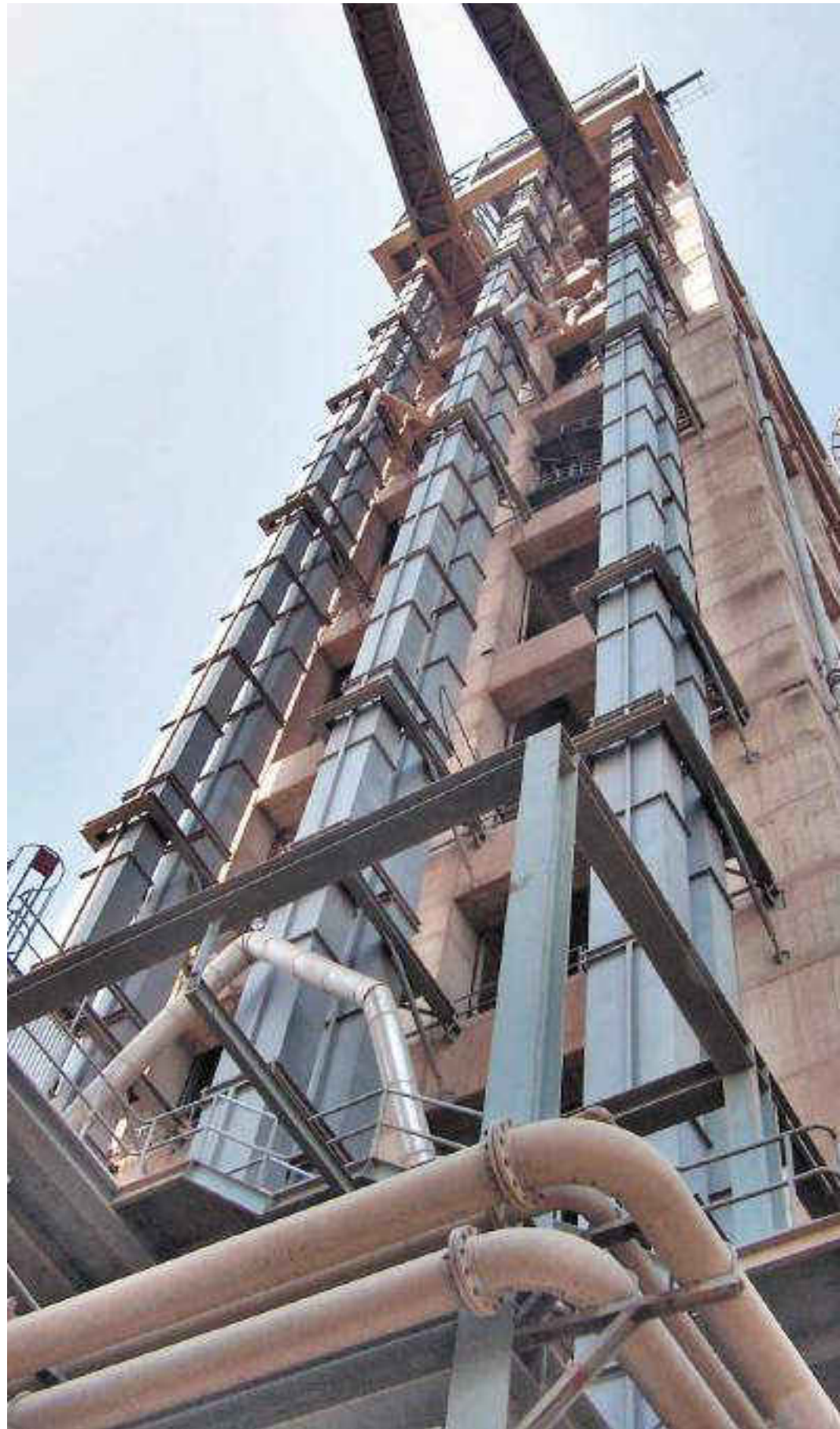
Belt Bucket Elevators handling raw meal
