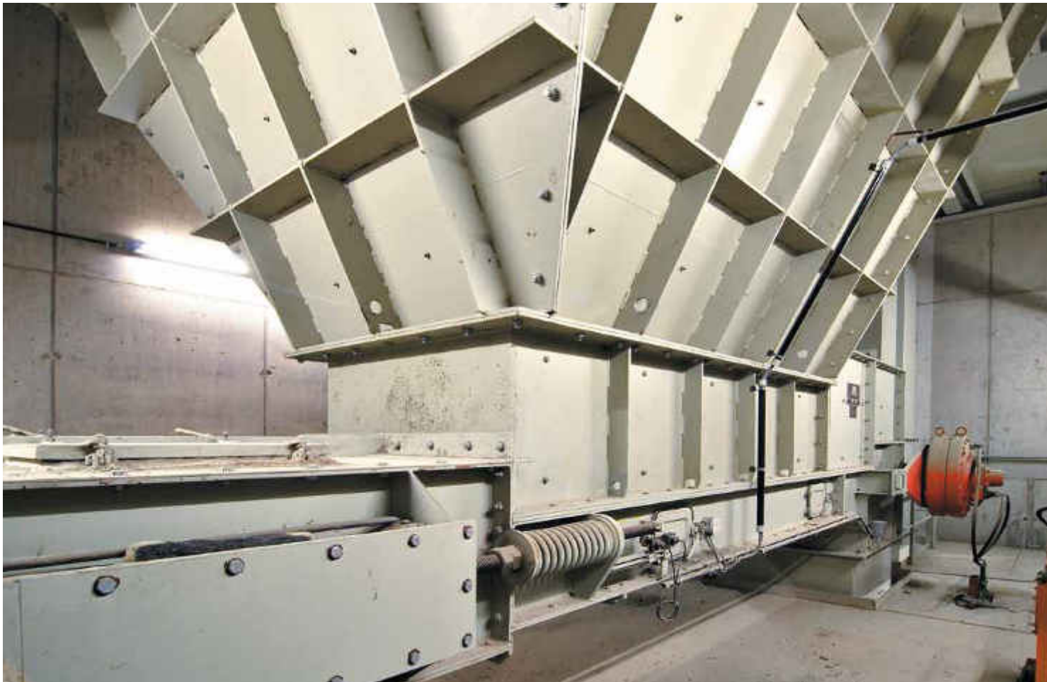
Hopper discharge with Armoured Chain Conveyor
