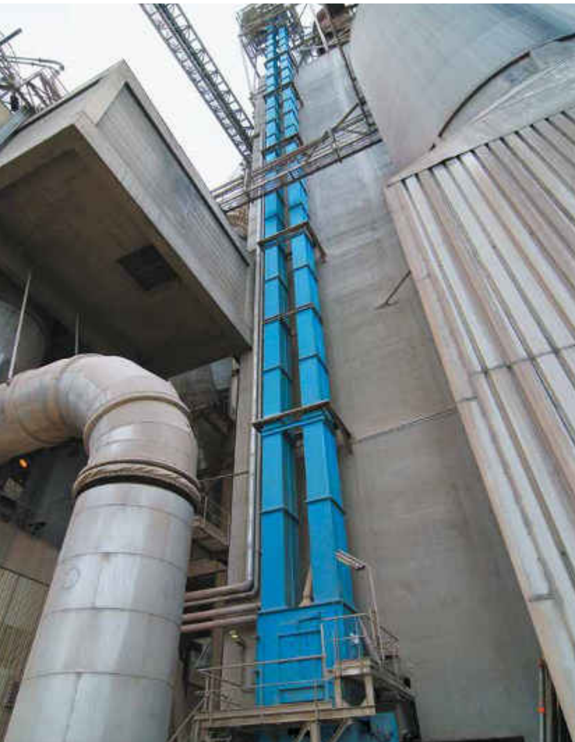
Bucket Elevator for silo feeding
