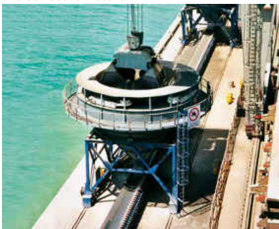
Unloading hoppers for clinker and additives
