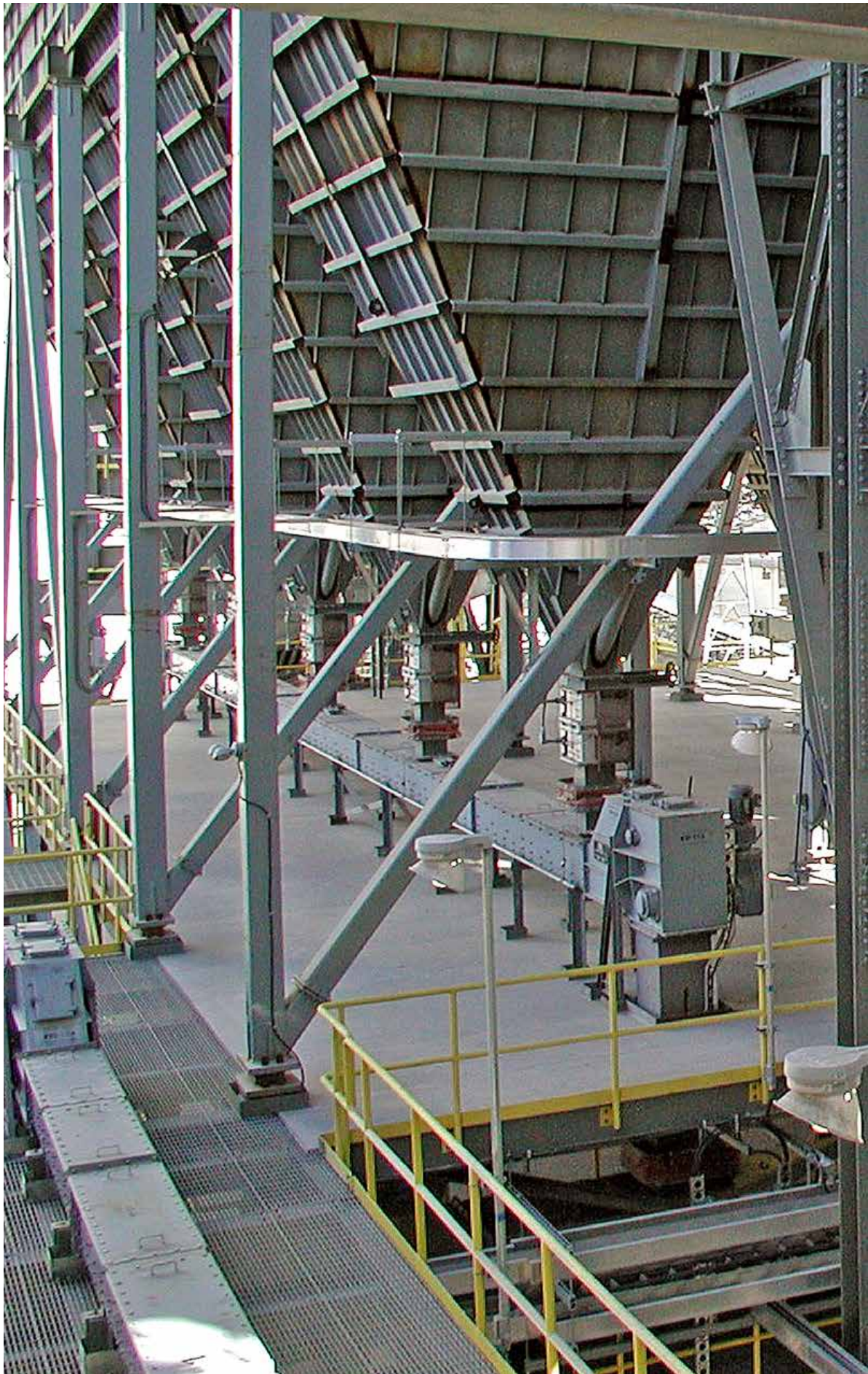
Filter dust reclaim
