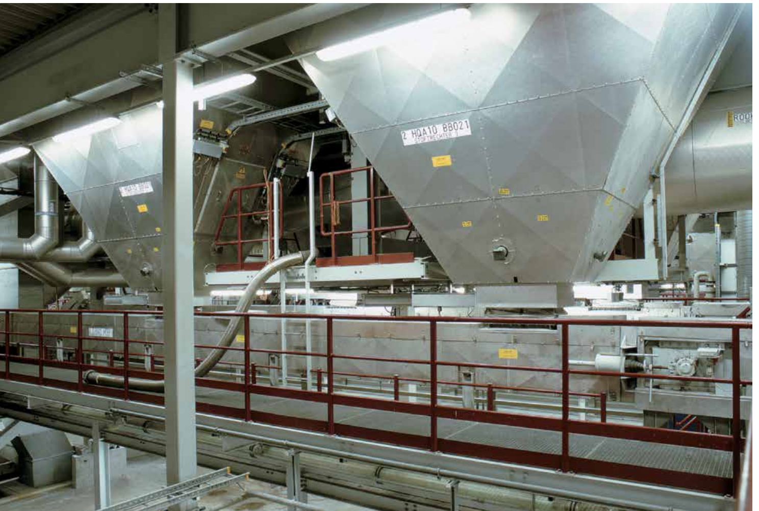
Hot boiler ash from a row of boilers
