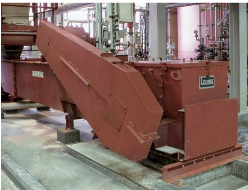
A double-strand chain conveyor loads FGD Gypsum from the flue-gas desulphurisation into the storage silo
