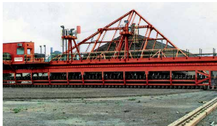
Bridge Scraper Reclaimer, 35 m span, 500 t/h, Iron Ore
