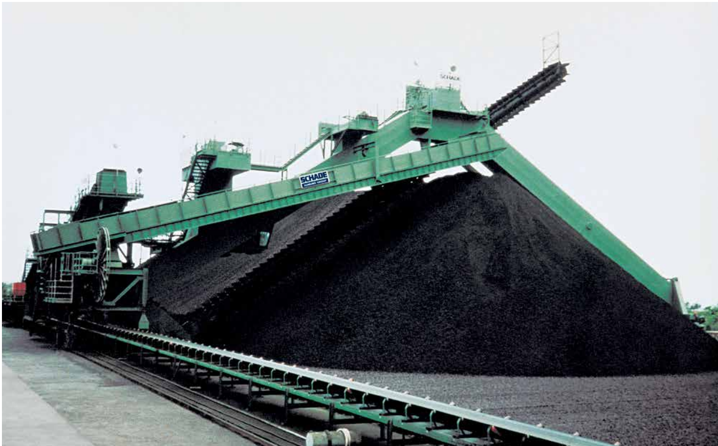
Combined Stacker Reclaimer, 46 m span, stacking 600t/h, reclaiming 300t/h, Coal
