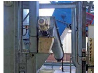
Discharge from Samson™ Material Feeder to Vertical Bucket Elevator
