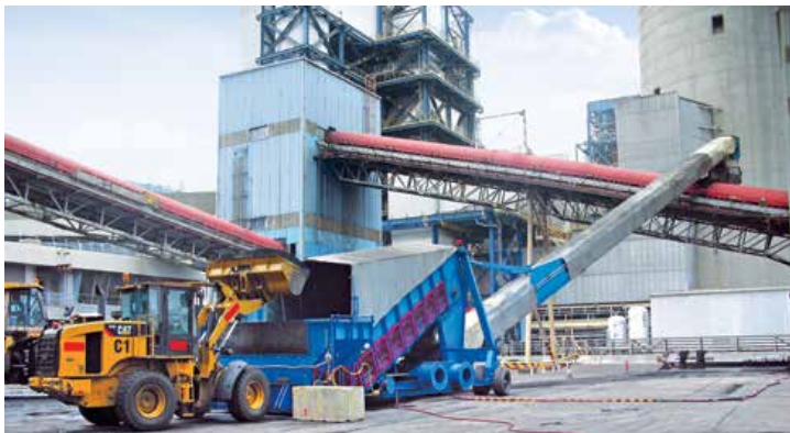
Stormmajor™ Boom Feeder introducing fuels to an existing conveyor belt at Hong Kong Electric
