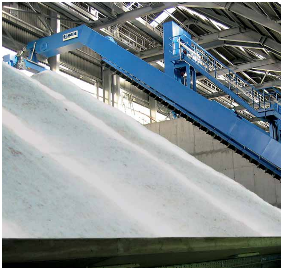
Portal Scraper Reclaimer
