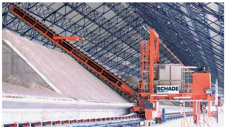
Cantilever Scraper Reclaimer
