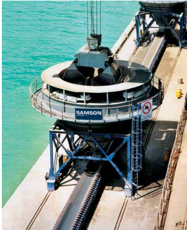
Ecological Unloading Hopper
