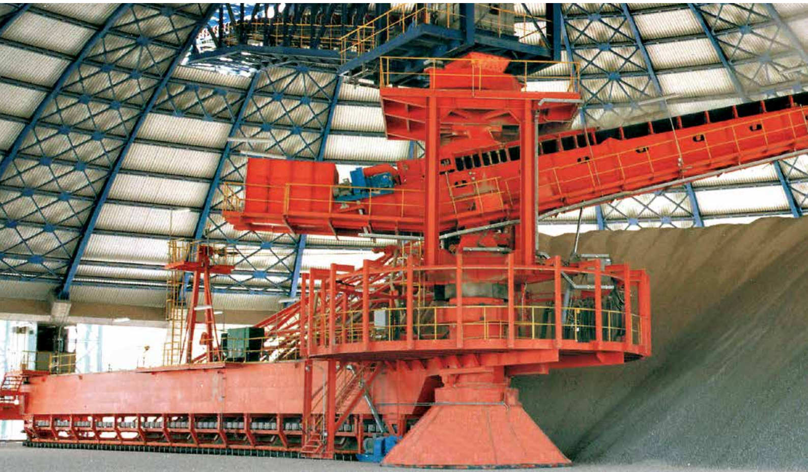
Circular Stacker with Bridge-type Reclaimer
