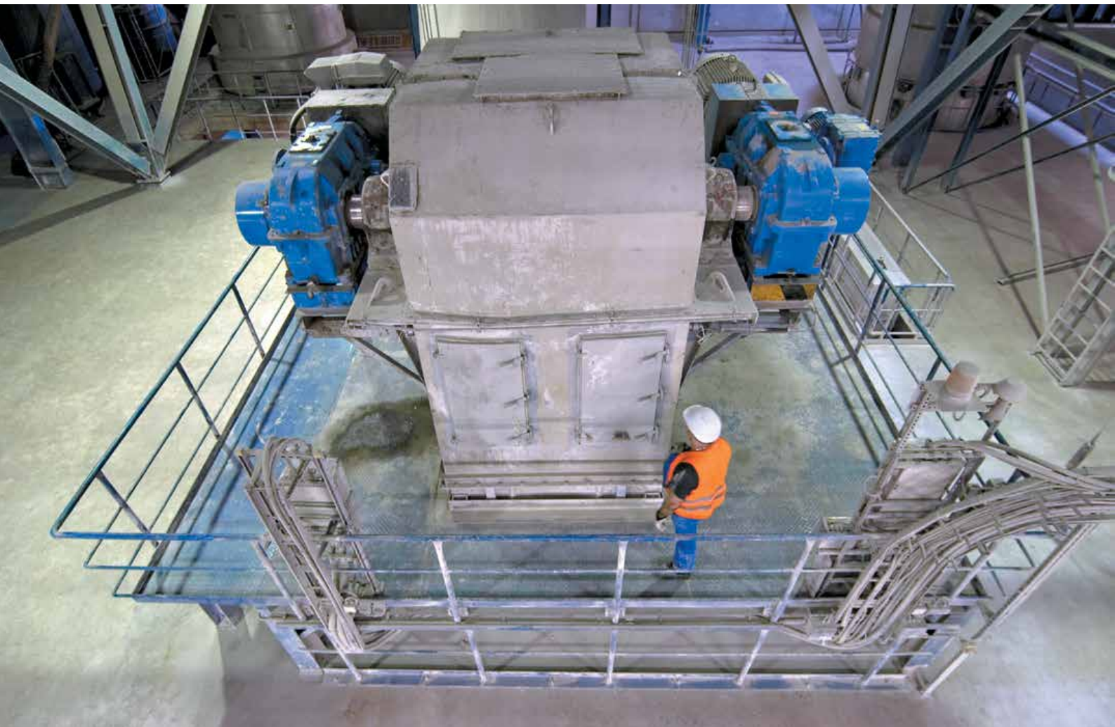
Head of Double Bucket Elevator
